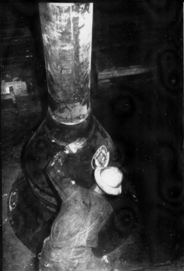
LOWERING THE 90-INCH diameter bit into shaft. Note drilling mud filling the shaft to top of cellar.
